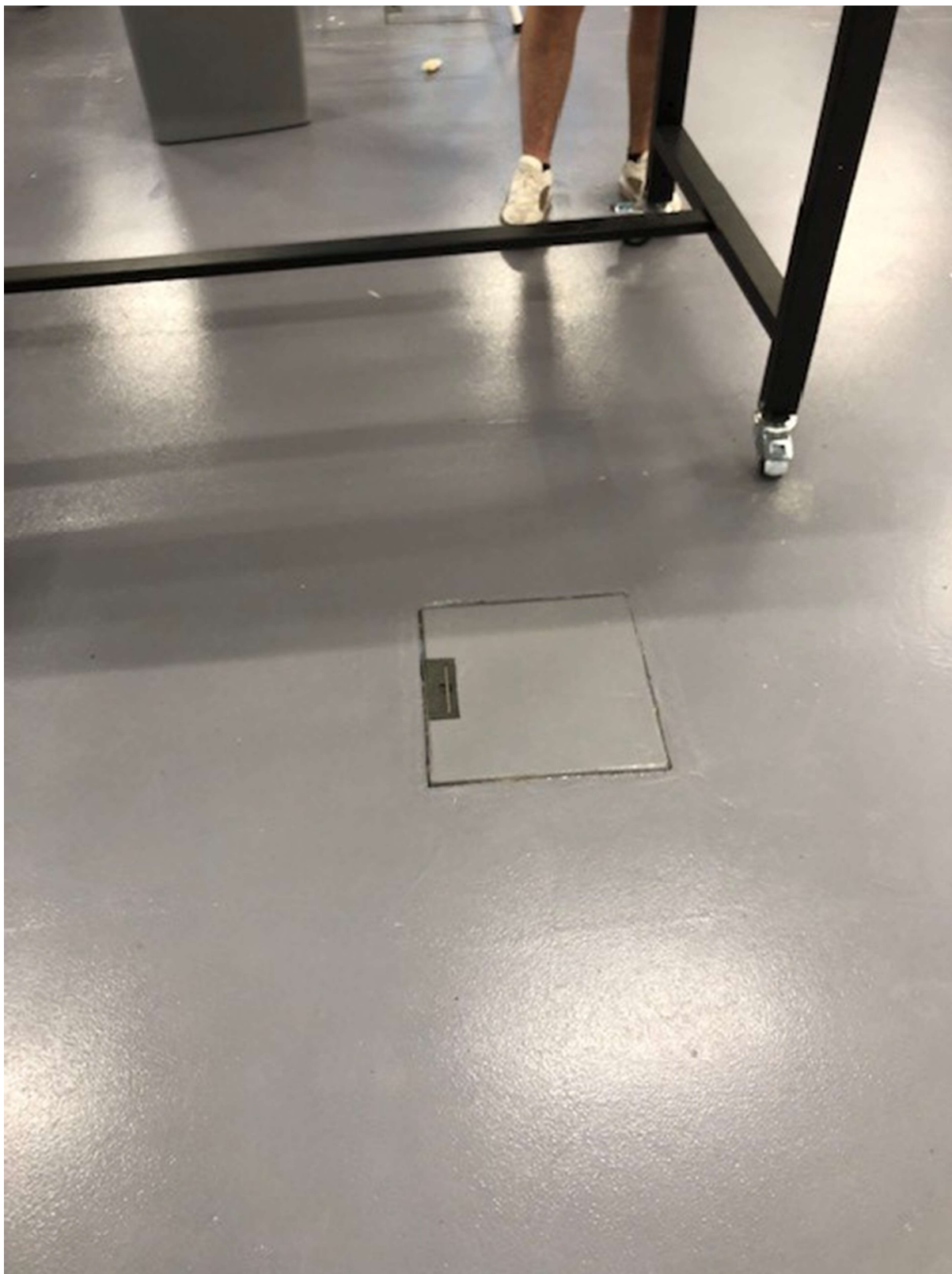
Photo 6 – Architect Laboratory Room showing electrical floor power outlet
