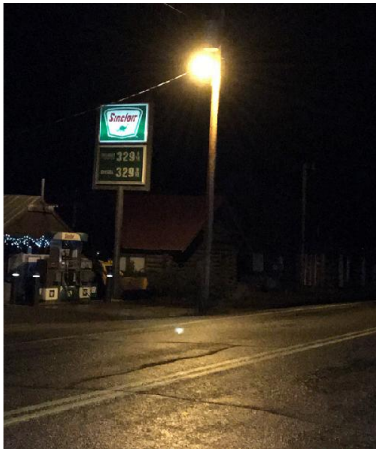
Figure 12: Sylvania 100 Watt, High Pressure Sodium, unshielded, 2100 Kelvin, 9500 lumens, in Stanley, Idaho. Installed pre-2012. Photo: Mayor of Stanley.
