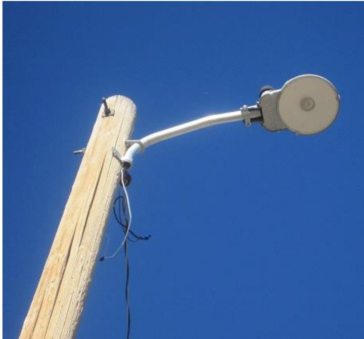
Figure 17: Daytime photograph of Evluma Areamax 3000 K LED fixture in Stanley, Idaho. 1 November, 2019. Photo: Jessica Heim.
