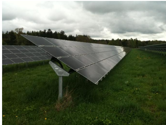
Figure 3 – Typical Solar Park
