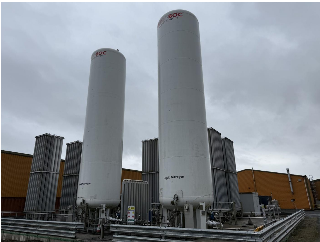
Figure 2 - BOC Liquid Nitrogen Gas Plant
