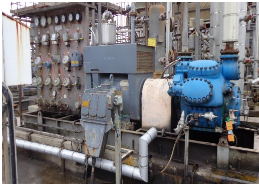
Figure 1: VRU Compressor and instrument panel
