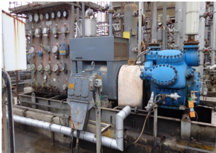
Figure 1: VRU Compressor and instrument panel
