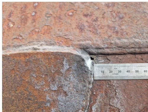
Figure 2: Localised through wall failure (Source: TATA Steel Internal Image)
