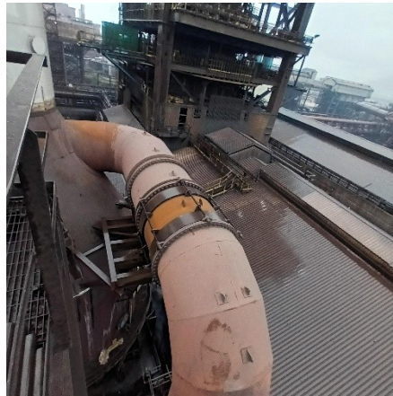
Figure 1: Crude Gas Main Column (Source: TATA Steel Internal Image)
