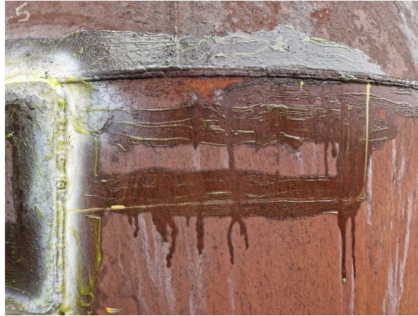
Figure 4 – Identified thinned area (Source: TATA Steel Internal Image)
