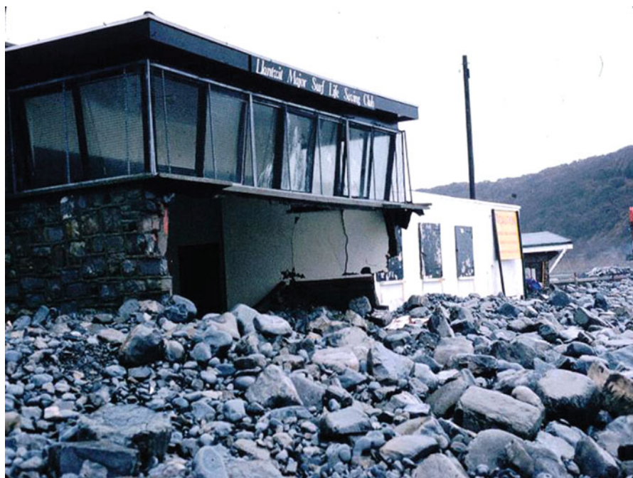
Fig. 17.2 Storm damage to Surf Life Saver Club
