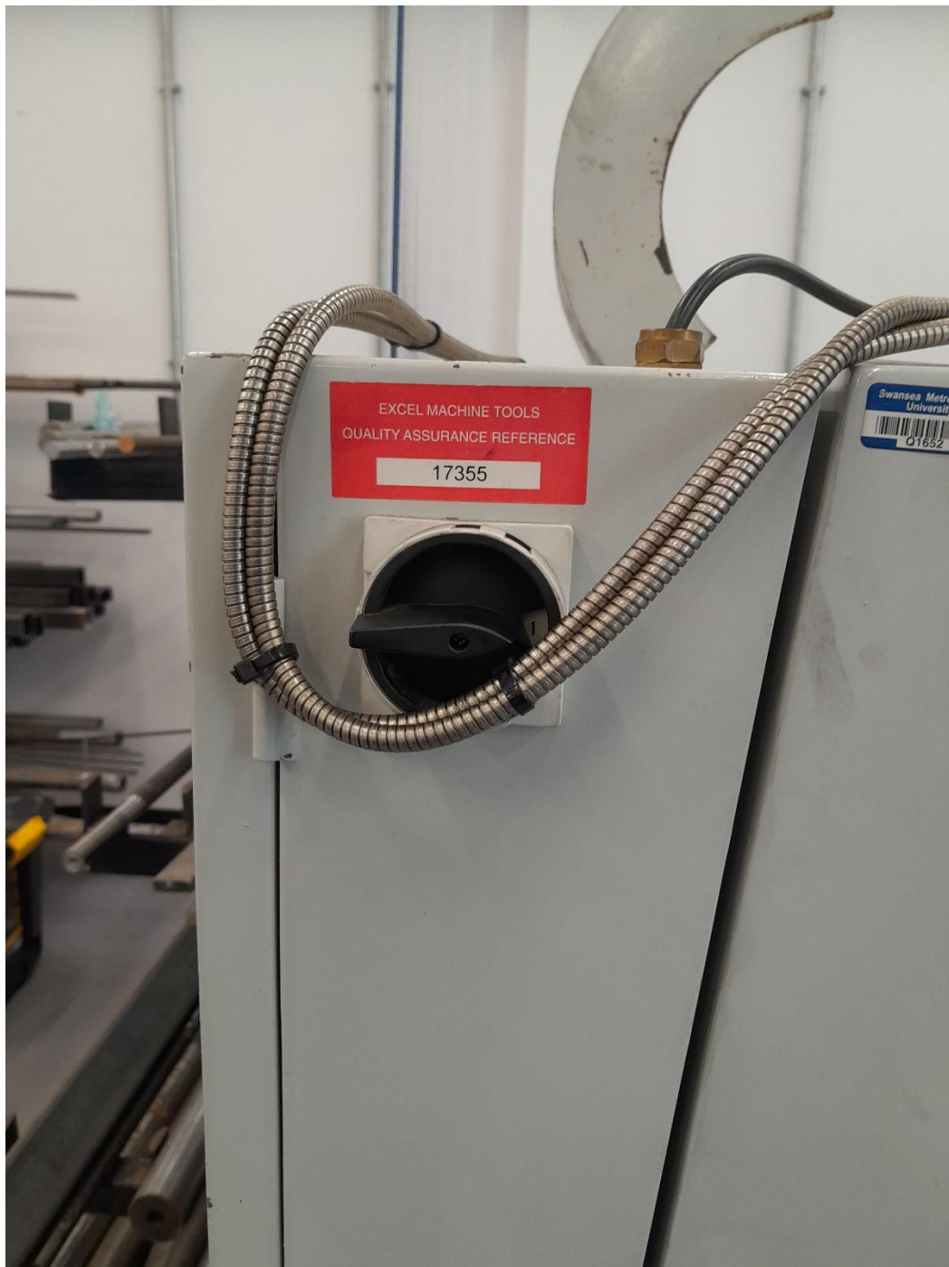
Figure 12: Power switch showing "on" position.
