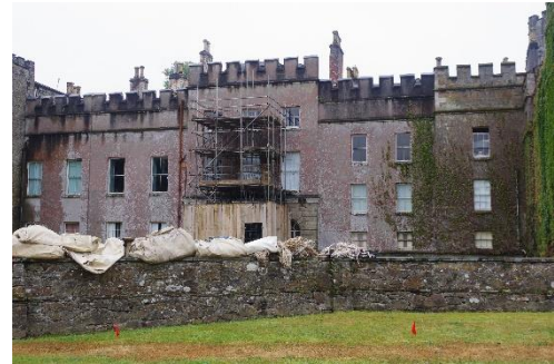
Figure 1 The front of Port Eliot, with the extent of the water damaged area indicated by the scaffolding © Cornwall Council.
