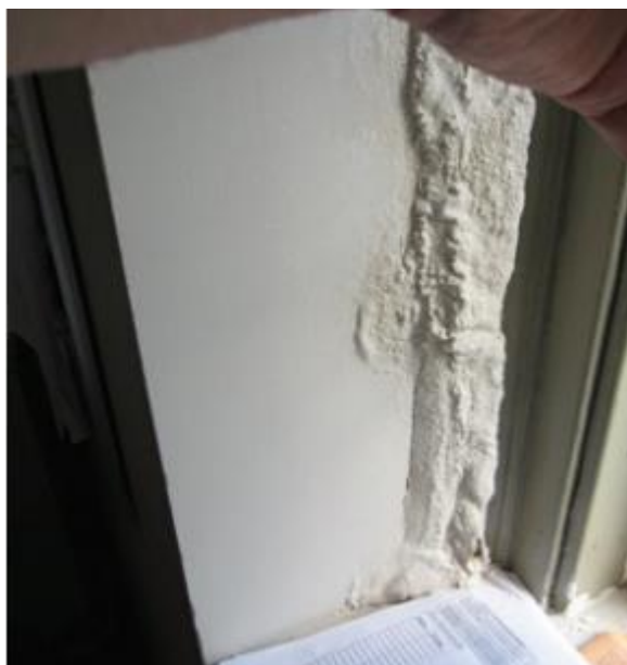
Figure 3.5 – Gypsum board Joint Damage
