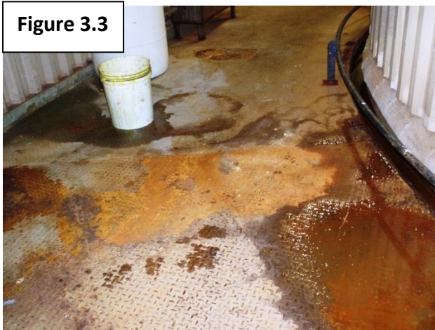
Figure 3.3 – Corrosion of floor
