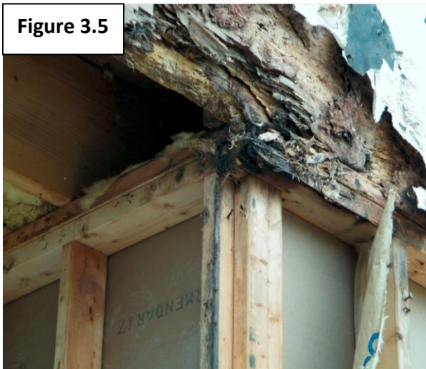
Figure 3.4 – Wood Rot due to water
