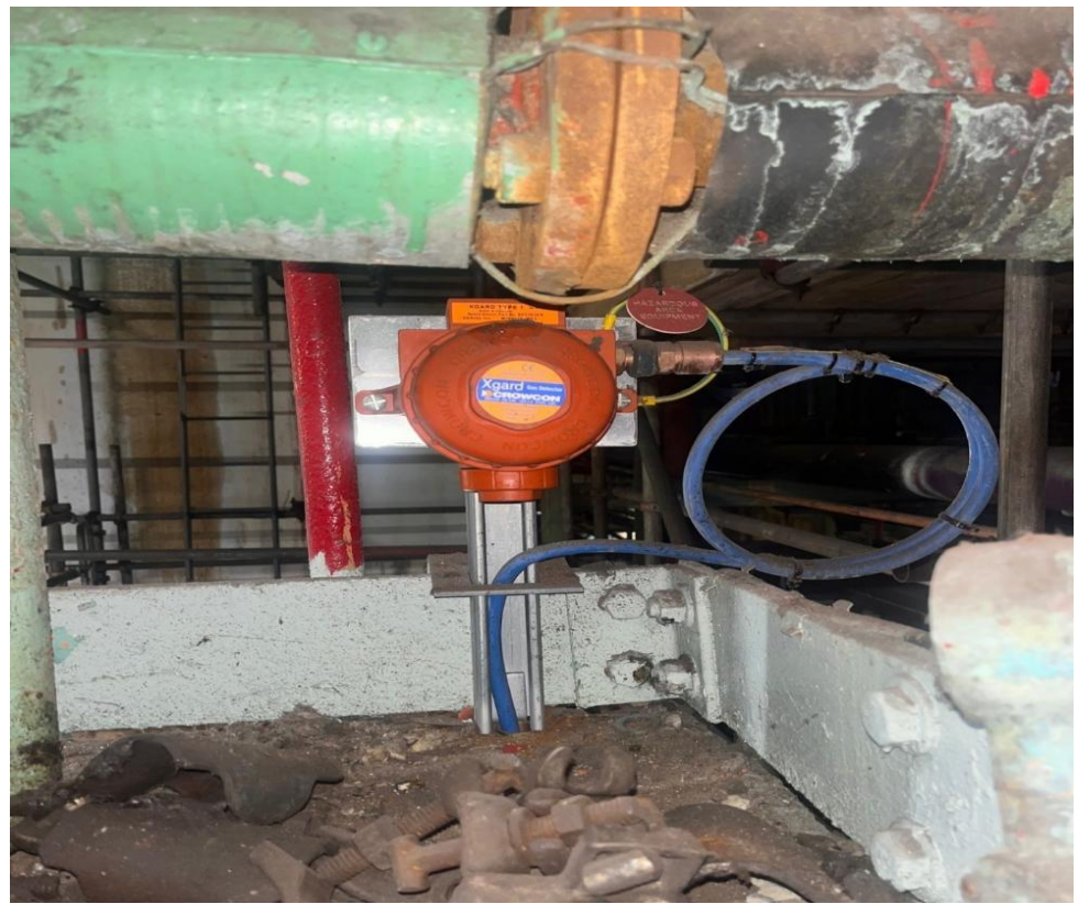
Figure.1: Crowcon Xgard Type 1 SO 2 detector installed within Kiln 1 activation area using low-level Unistrut mounting arrangement.
