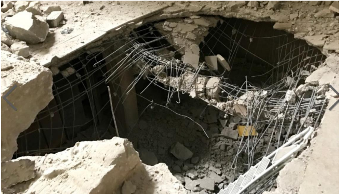
Fig 10: The large hole in the floor of the museum, a result of ISIS using explosives to access archives (Wedeman 2017).
