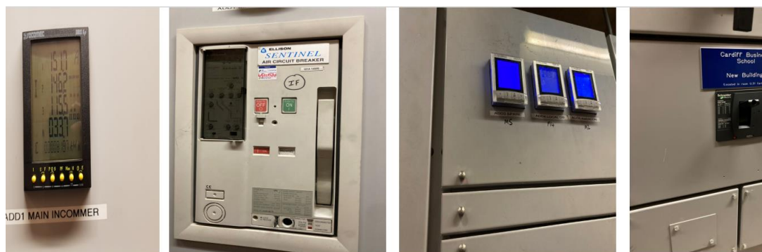
Figure 9 Energy consumption meters at the building
