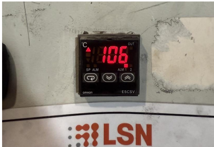
Figure 8 – PLC controlled thermostat not allowing powder release until set temperature is met.
