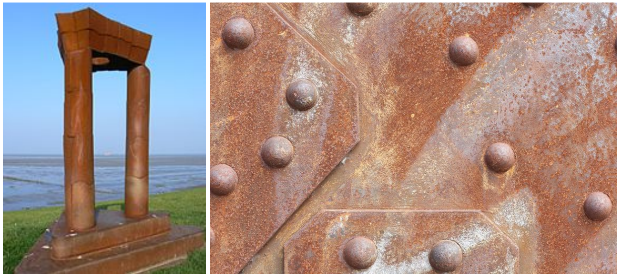
Figure 8: Light rust formation which acts as protection allowing the structure to retain its structural properties (Gräfen, Horn, ESchlecker, & Schindler, 2000)
