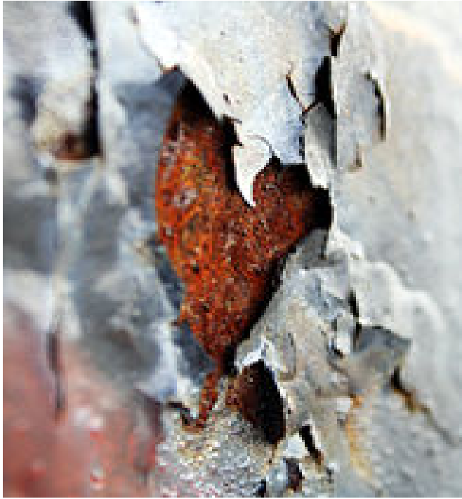
Figure 9: Flaking coating exposing sections of the iron surface to rust
