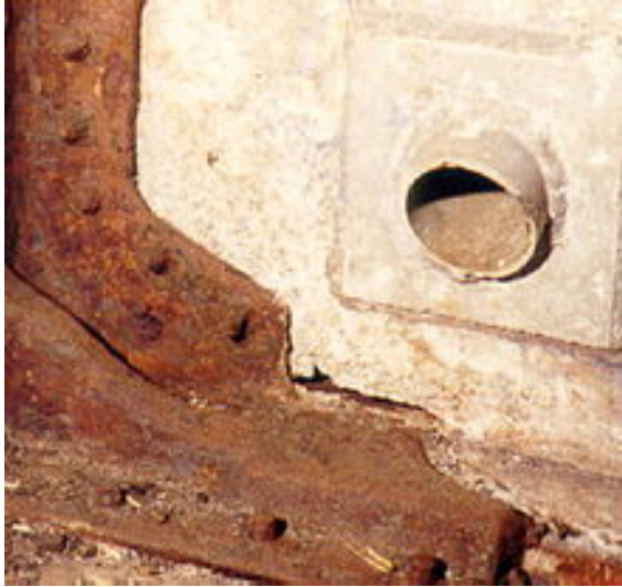
Figure 4: Galvanic corrosion (Gretchen, 2015)
