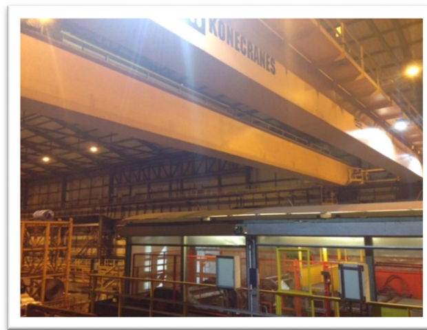
Figure 4 - CAPL overhead bridge crane
