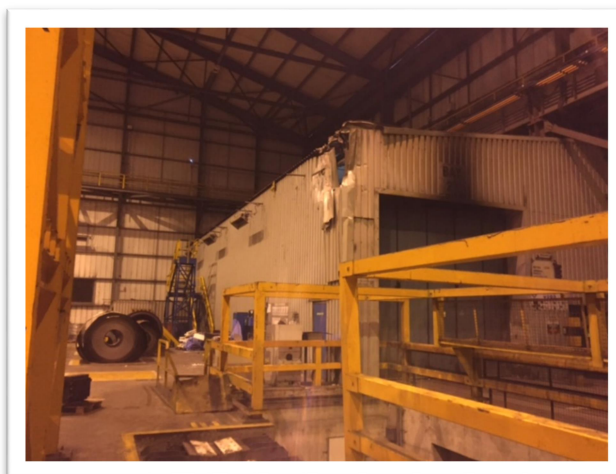
Figure 1 - Damage to infrastructure from crane collision in CAPL
