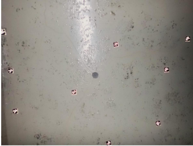
Figure 4, Core Sample Cracking in Room 2 (taken with digital camera)
