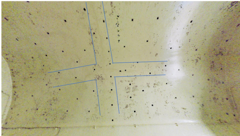
Figure 3, Cracking in Room 1 (taken from 3D Scan)
