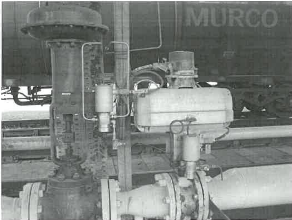
Figure 1 – illustrates the SIS (Safety Instrumented System) shutdown valve and actuator.
