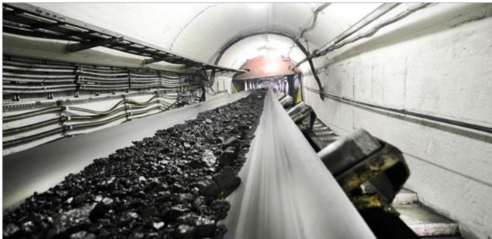
Figure 4 - Coal Conveyor Belt
