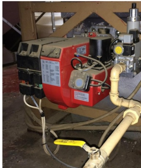
Figure 6: The gas system including the solenoid and ignitor connected to the roasting drum.
