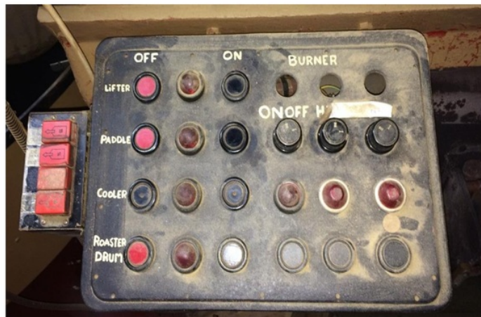
Figure 5: The existing control console.
