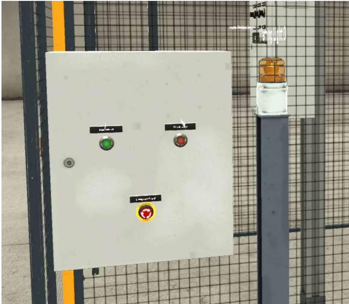
Figure 86 - Main control panel
