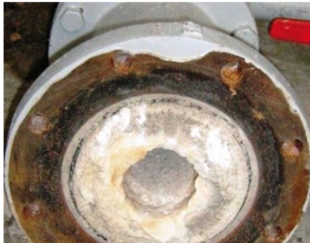
Figure 4 - Shell and Tube heat Exchanger - Chemical Fouling - [16]
