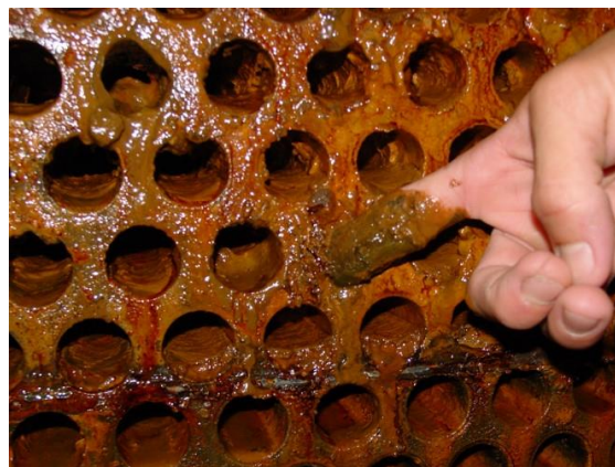
Figure 6 - Shell and Tube Heat Exchanger - Biological Fouling - [26]
