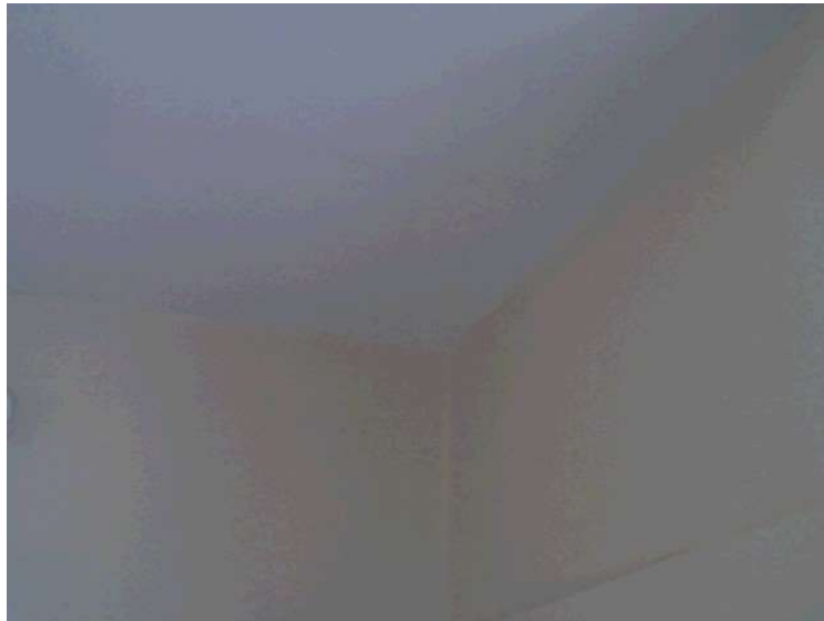
Figure 3.2.1: Internal image external Wall Corner (Author, 2018)
