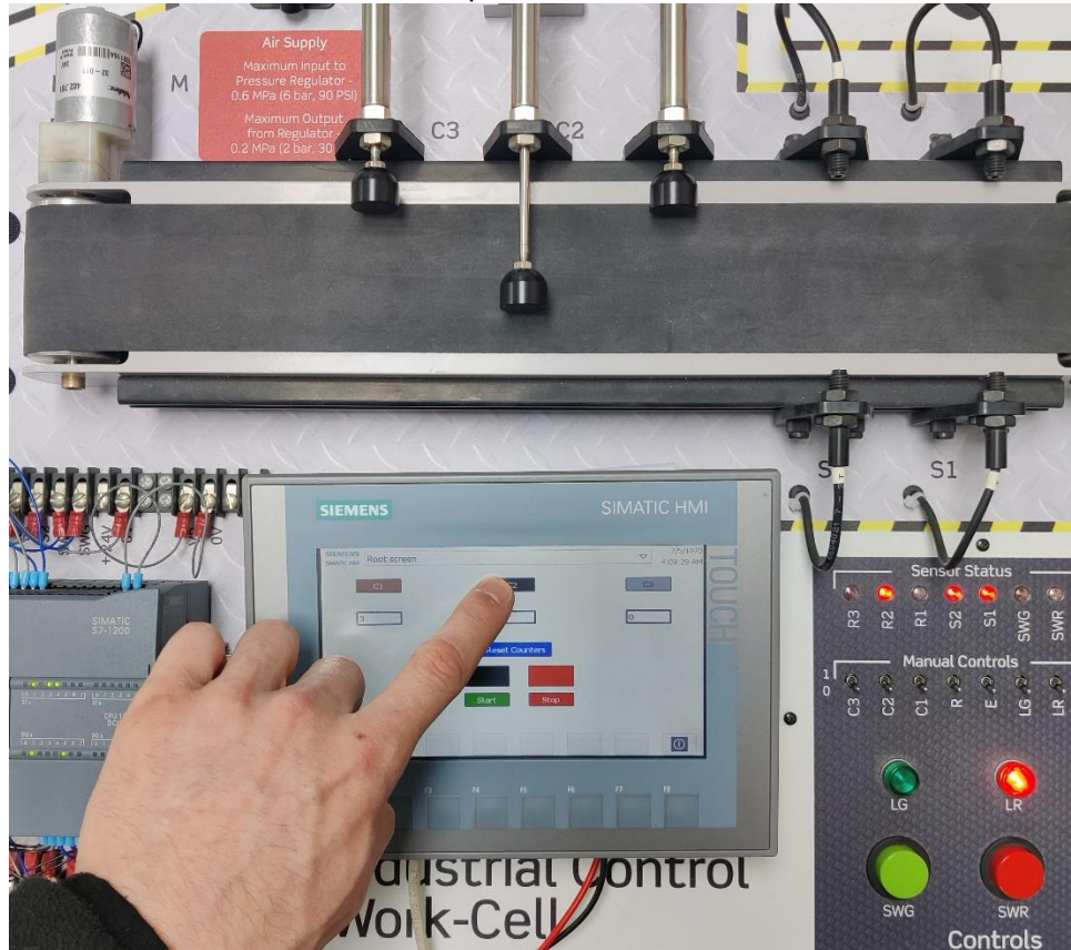
C2 in manual operation for maintenance.
