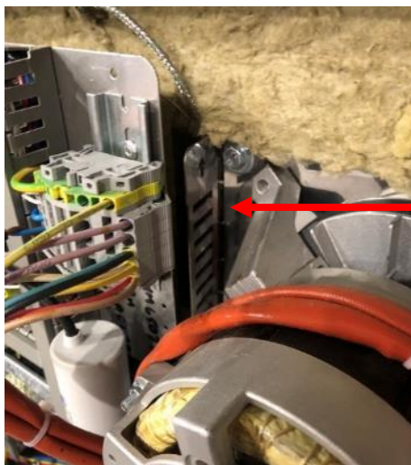
Figure 30: Electrical Panel Brace
