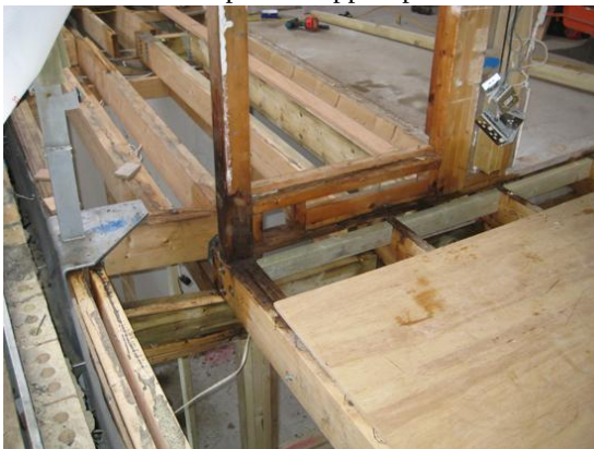
Figure 1: Remedial work in progress to a TF building. The vertical load from the post in the centre of the picture was supposed to be transferred by a set of site-fixed studs below (now installed) but these were originally missing. The resultant distortion of the frame led to severe water penetration from a balcony. (© Watts Group/Trevor Rushton) The design was fully detailed by designers and required 'loose studs' to be inserted within certain internal wall panels to increase the load-bearing capacity of the panels to support point loads from the roof structure. The building was clad in brickwork.
