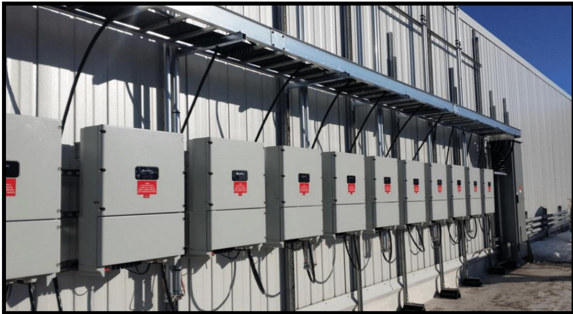
Figure 19: Array of String Inverters. (Greentech Renewables, 2025)
