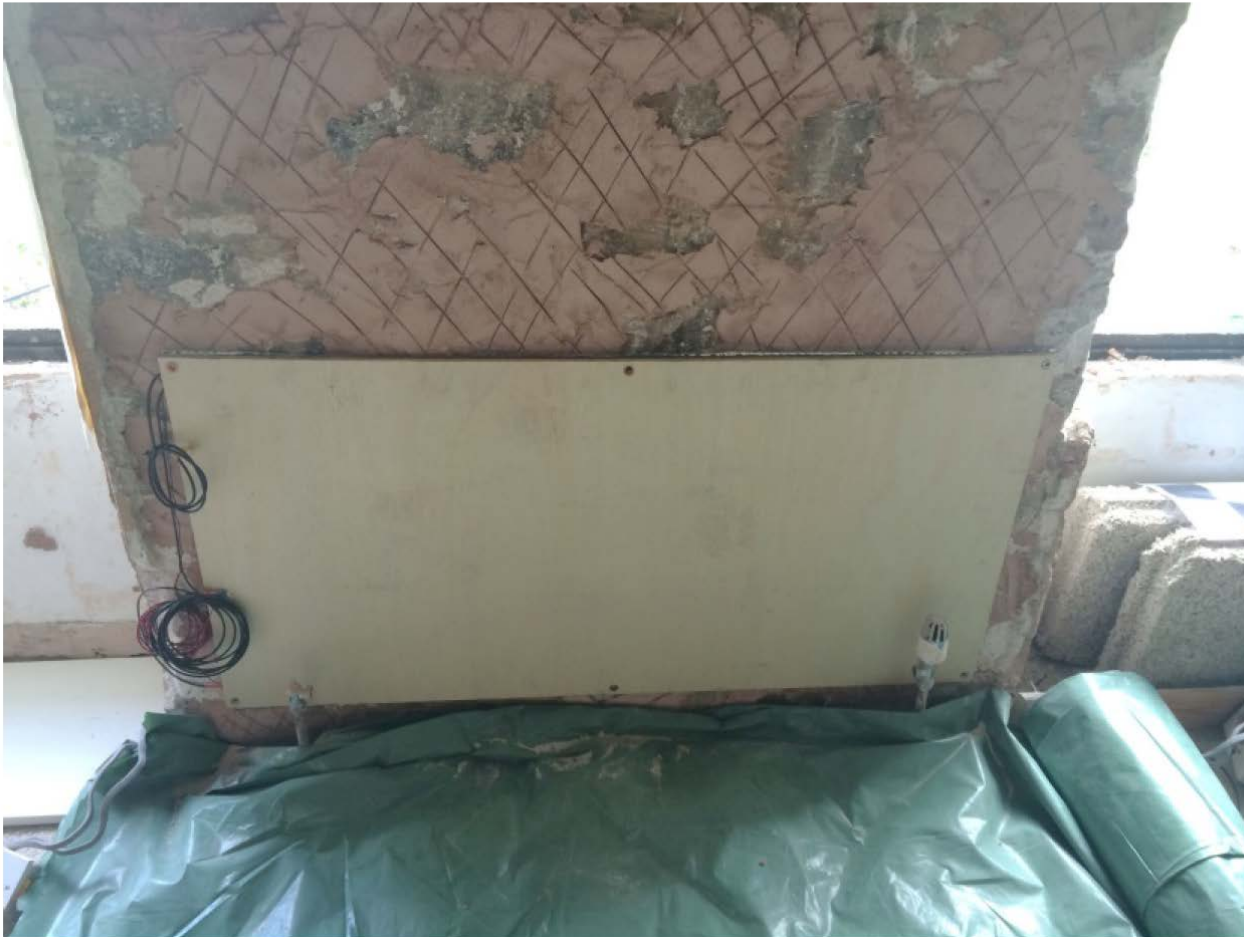
FIGURE 6 showing gap at top of panel two
