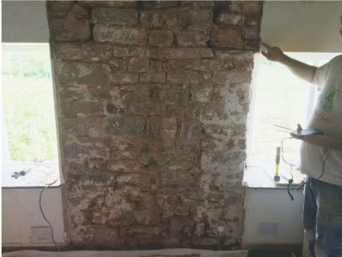
Central section between windows with existing plaster removed. Gary Perkins is pointing to the upper right hand side where the stonework is poor quality and large voids are evident. Moisture content readings are taken.
