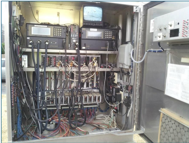
Figure 3: A traffic control cabinet coming in the north American flavour.[14] The specific makes and models of the equipment can and does differ from country to country, but the general layout is common.
