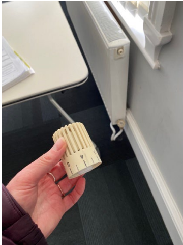
Figure 2: Broken radiator valve (Parnaby, 2026).
