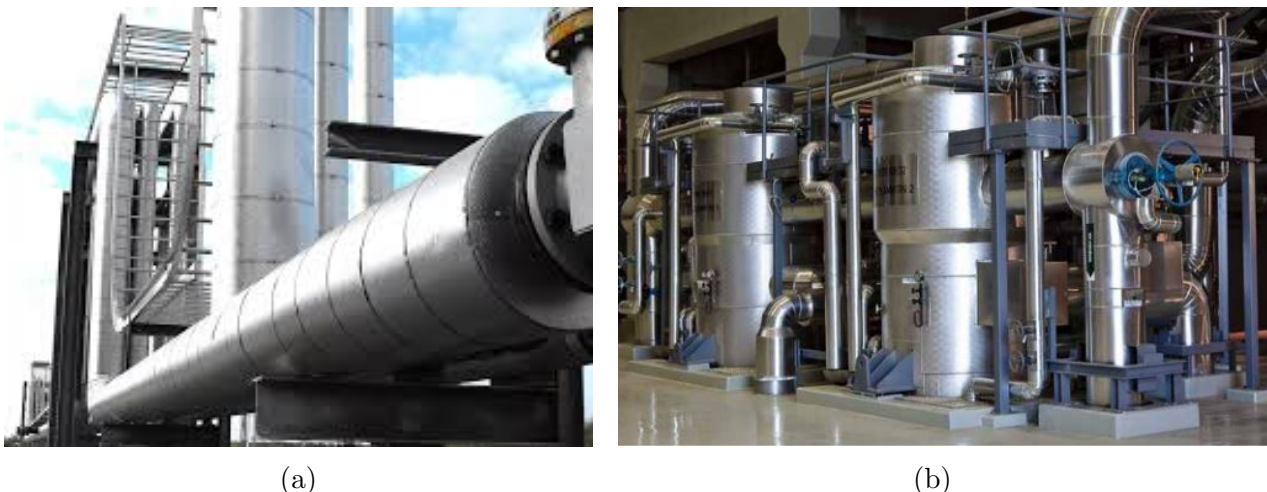
Figure 2.2: a) Insulated pipework and b) Insulated vessels
