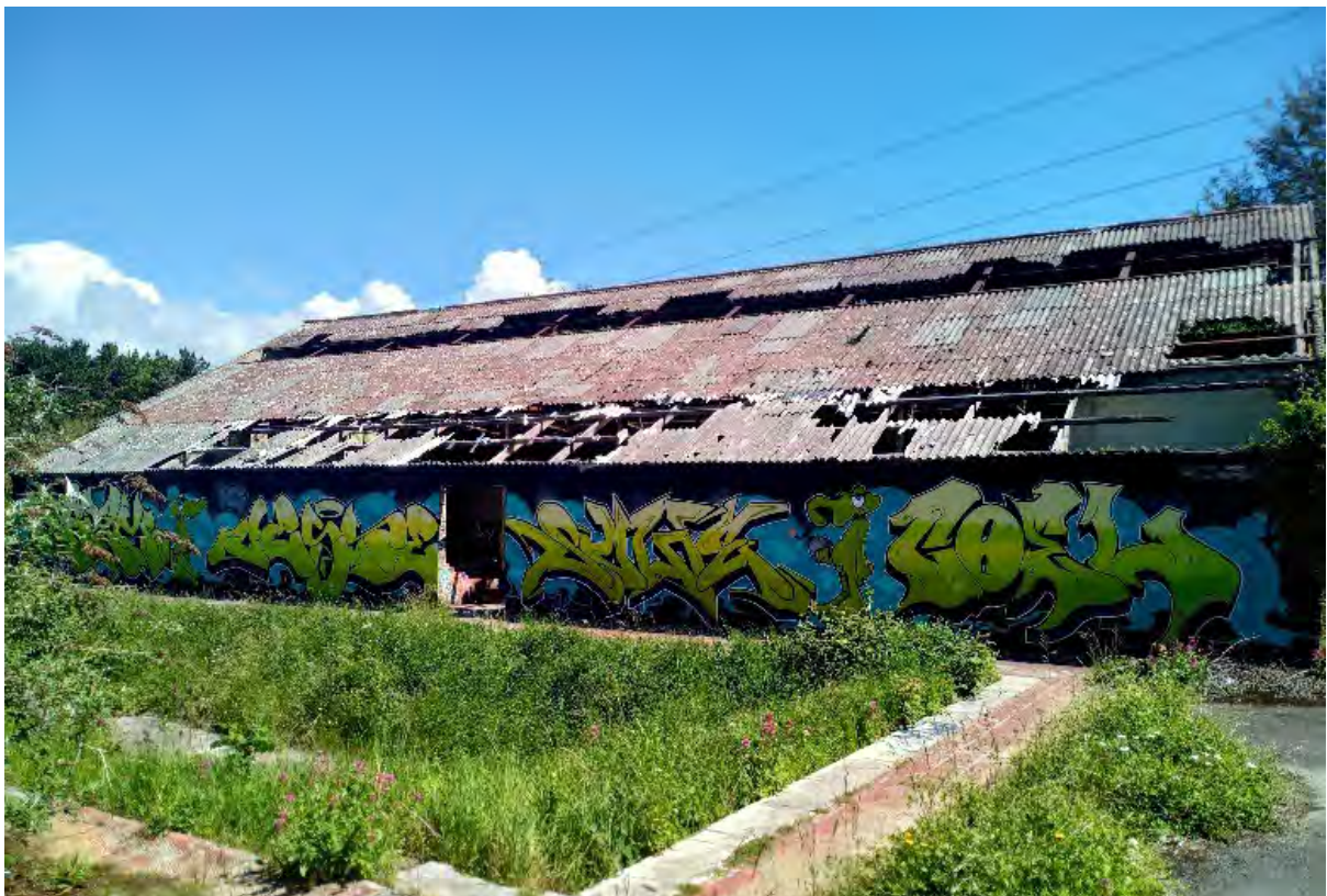
Figure 42 – Gymnasium with natural decay of the roof structure along with the swimming pool in the foreground (Author, 2021)
