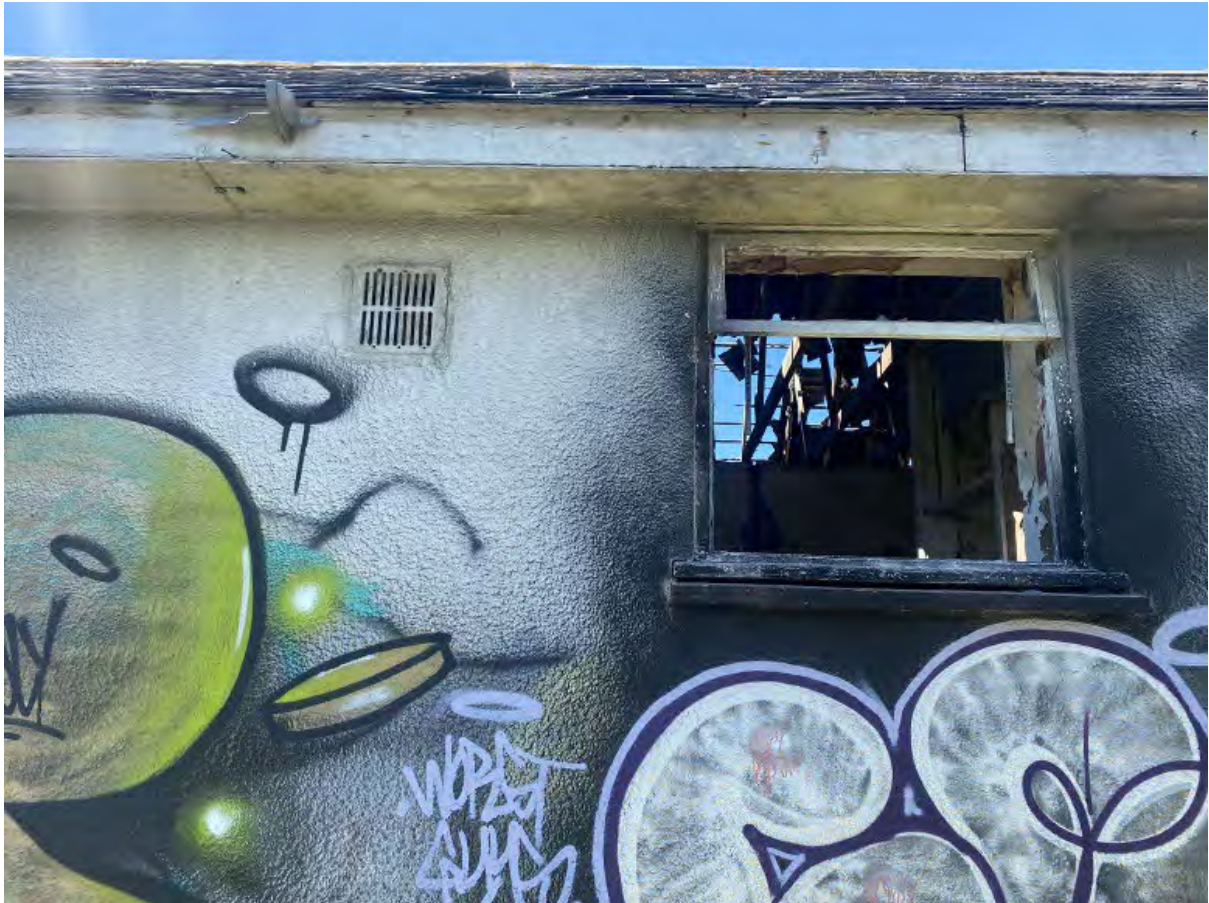
Figure 41 – Evidence of fire spread in one of the classrooms (Author, 2021)
