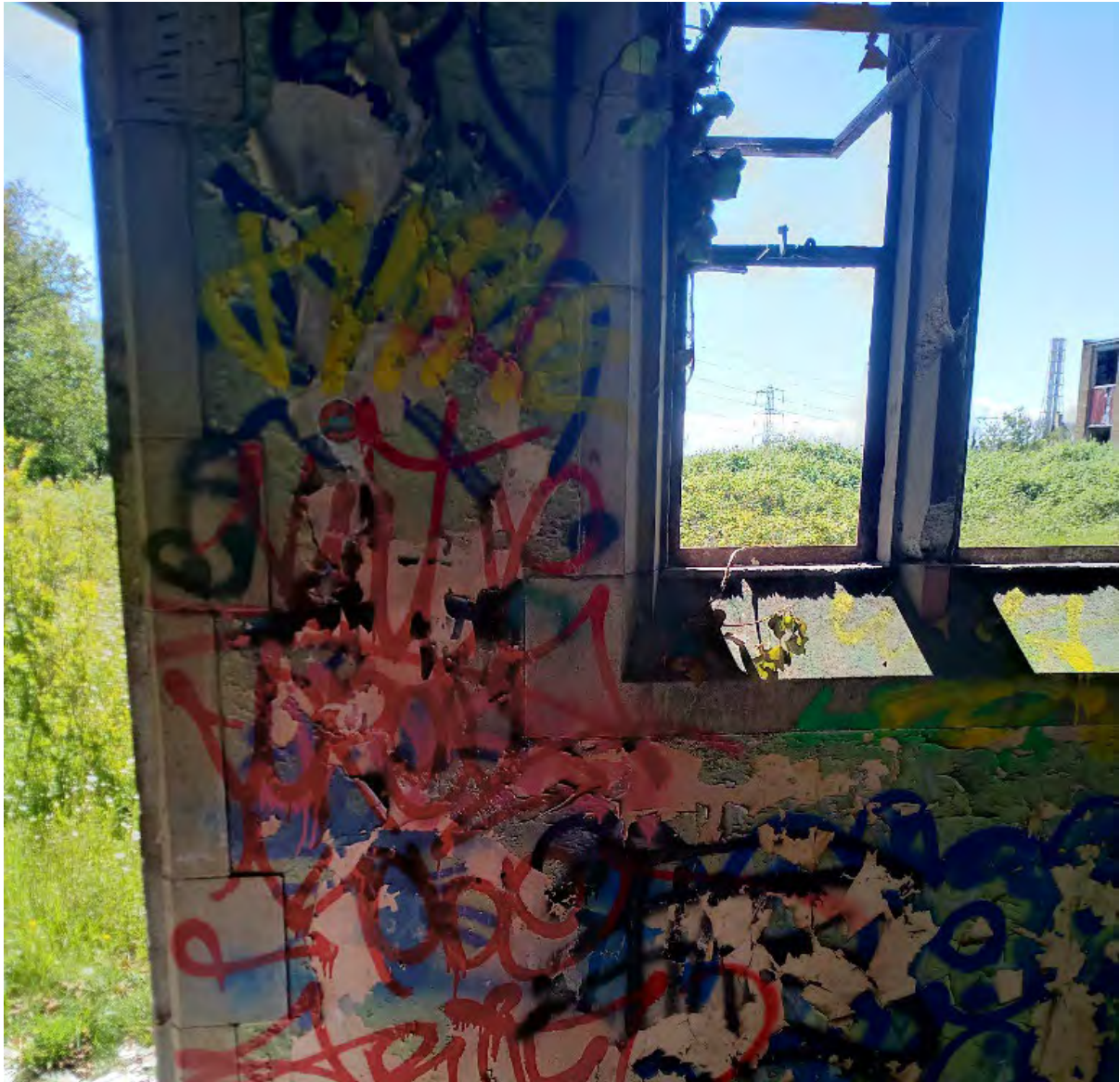
Figure 40 – Graffiti plastered on this wall in the chapel (Author, 2021)
