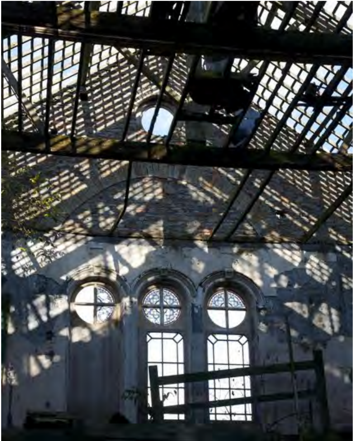
Figure 52 – Interior of Bethania Chapel in 2009, falling into disrepair (Whitmore, 2009)
