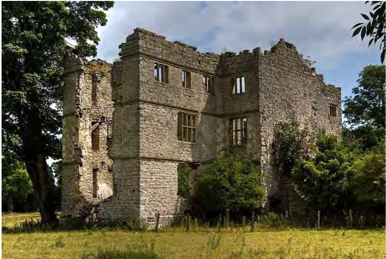
Figure 62 – Exterior of Foxhall Newydd falling apart (Searle, 2014)
