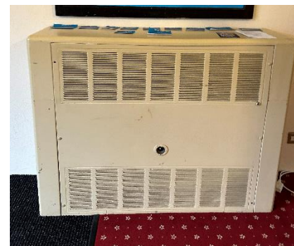
Figure 8 Showing Radiators- Author
