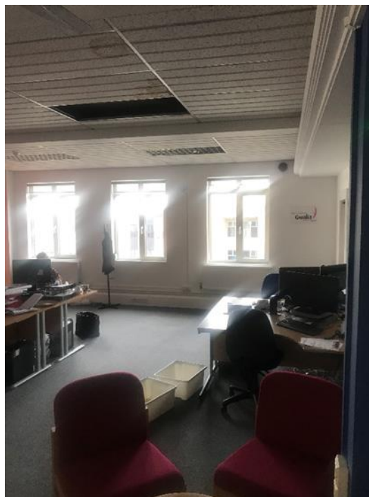
Plate 10: Showing staining from water ingress on roof
