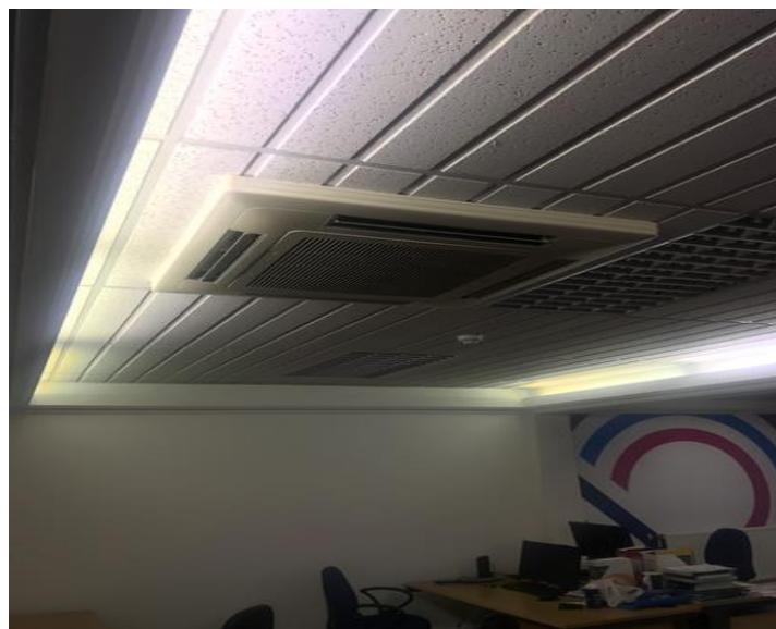
Plate 15: Ad-hoc Air condition ceiling cassette
