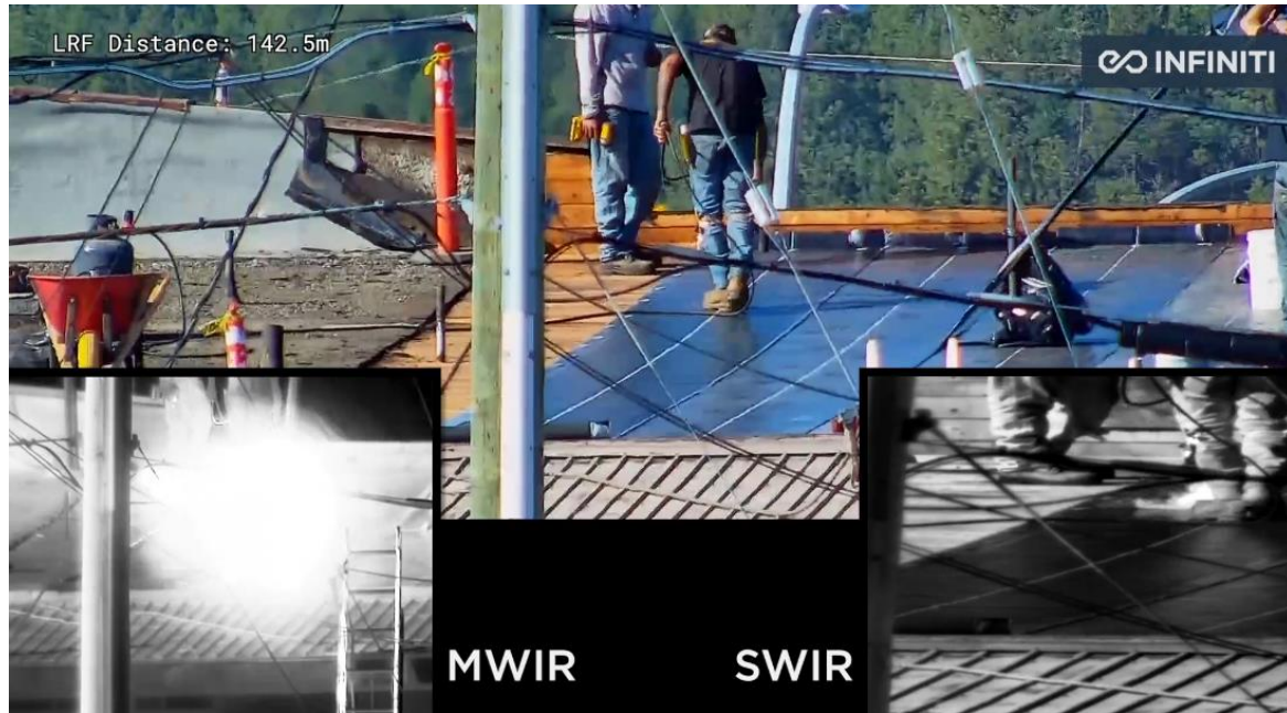
Figure 8: A scene showing workers using a heat gun on a roof recorded in visible (centre) MWIR (left) and SWIR (right) [7]
