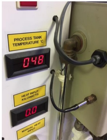
Figure 5. Heater tank level and temperature sensors
