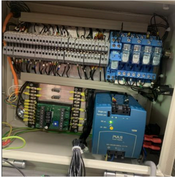
Figure 81 Internal panel wiring
