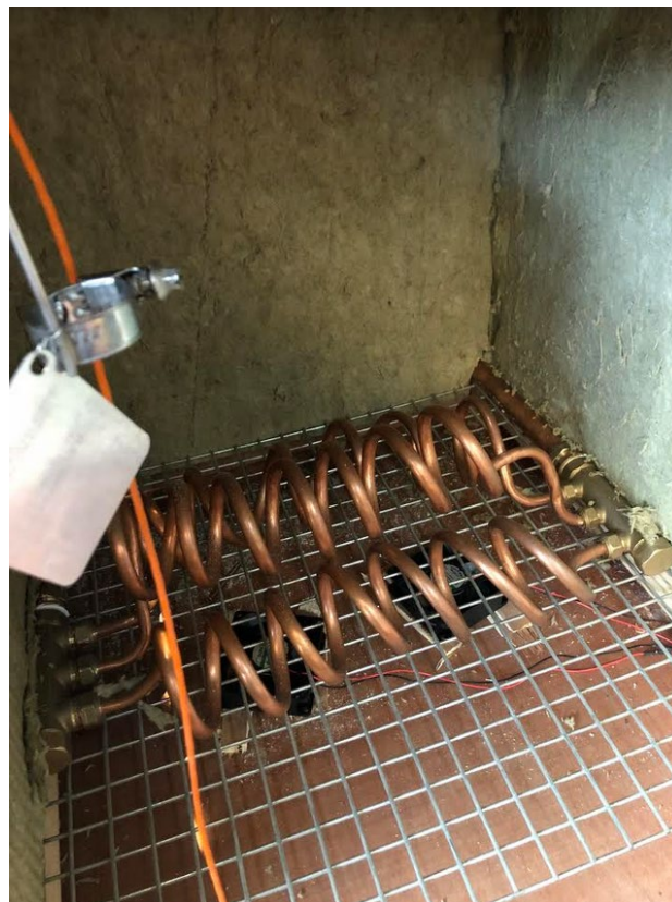
Figure 56 - Copper Coils used for heating the Room.
