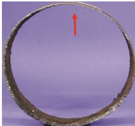
Figure 13: Example of Internal Corrosion
