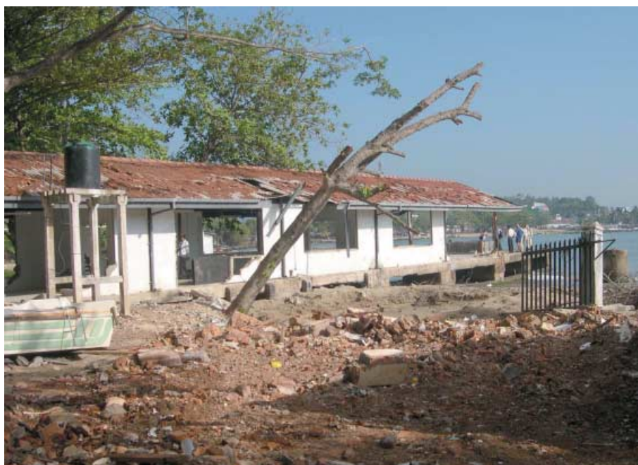
Figure 19. The MAU headquarters destroyed by the tsunami on 26 December 2004. (Avondster-Project)
