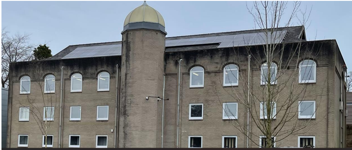
Photo showing PV modules installed on roof.
