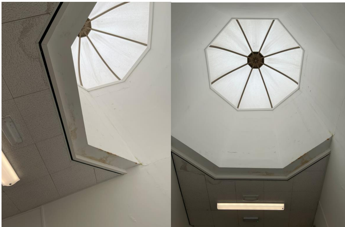
Photo showing condensation around ceiling. (own image, 2024)
