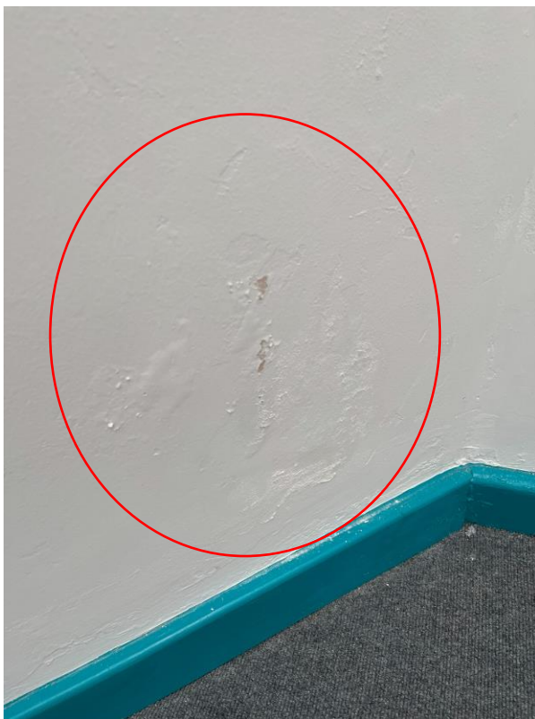
Photo showing dampness in wall below the cupola. (own image, 2024)
