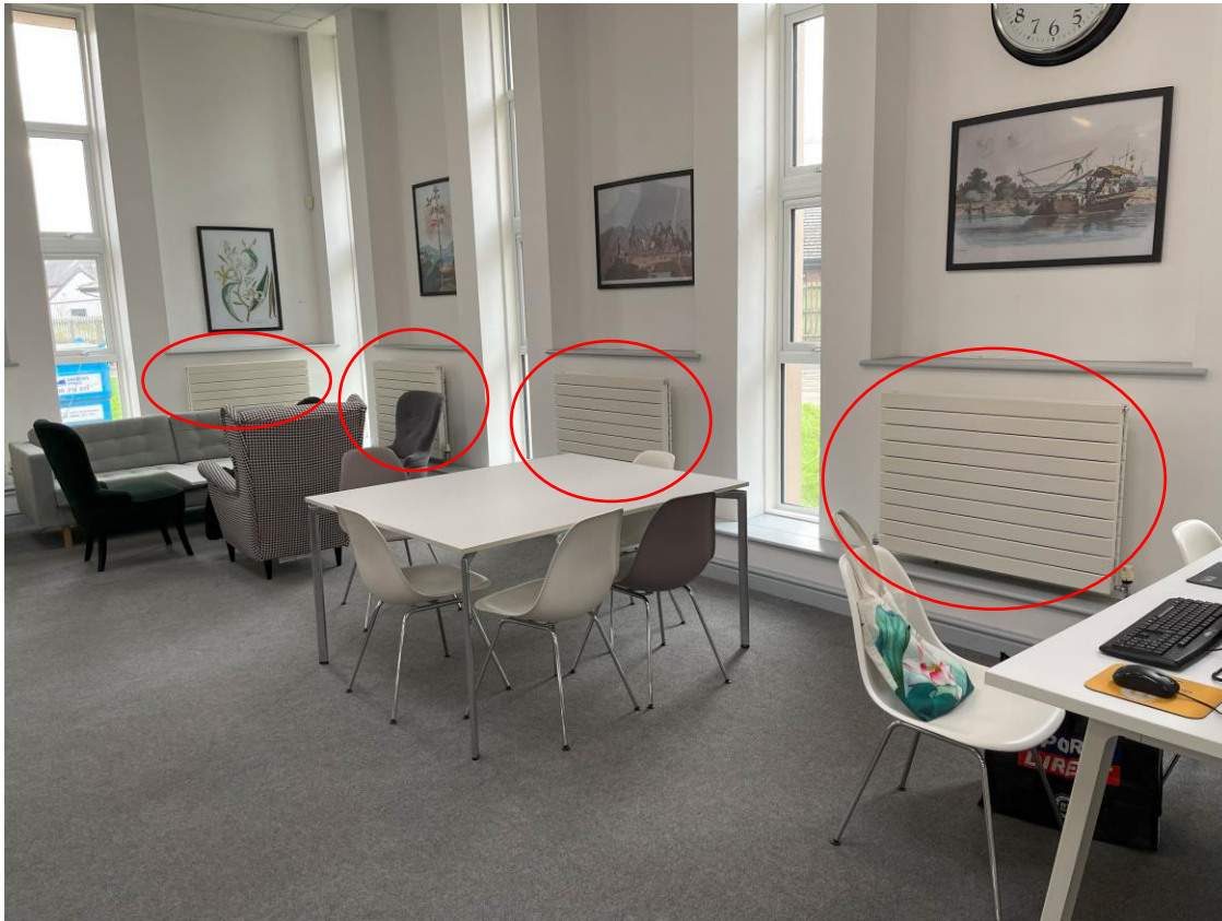
Photo showing heaters around the reading room (own image, 2024)
