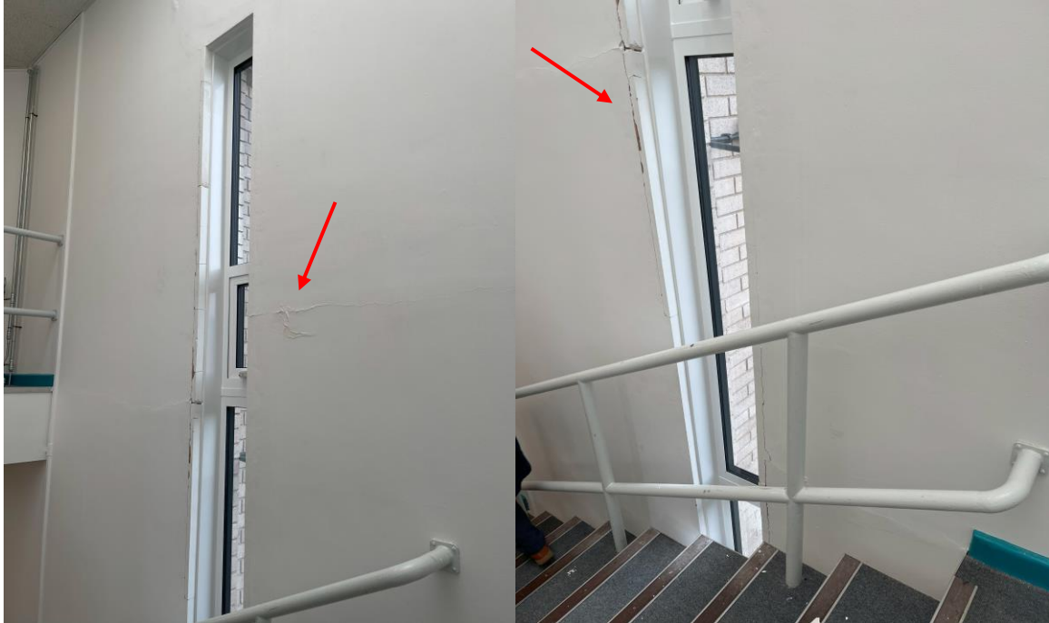
Photo showing cracks along the walls below the cupola. (own image, 2024)
