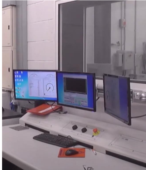
Figure 5 (control panel where dyno is operated behind safety glass)
