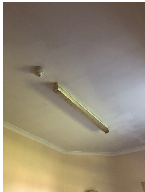
Figure 2: Example of Fluorescent Lighting
