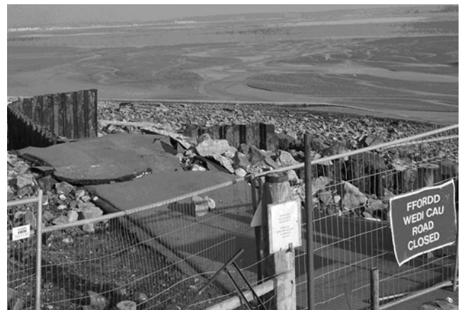
Figure 4. Coastal path failure
