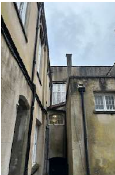
Figure 8 Showing External 'Stucco' technique with added modern materials which will be required to be removed, traditional lime-based material reapplied.
