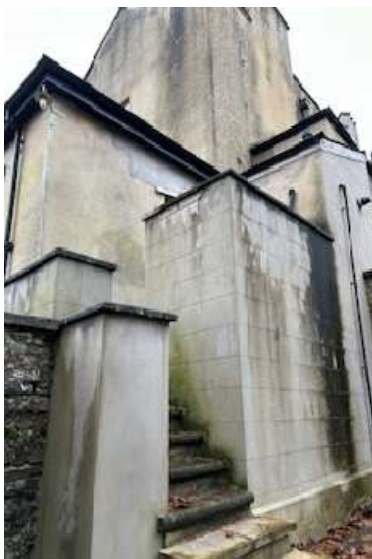
Figure 9 Showing modern repair work that will require attention furthermore applying traditional lime-based render instead.
