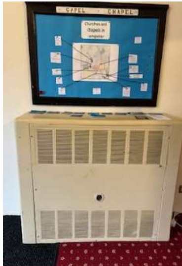
Figure 7 Showing current heating strategies which is gas mains fed, conventional stand-alone system.
