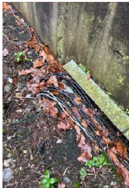
Figure 5- Showing external wiring around building
