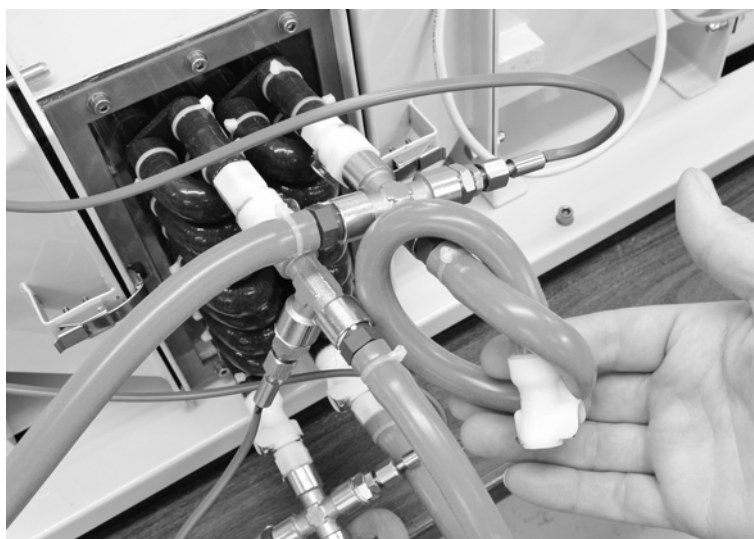
Figure 32 Some Pipe Connections are Not Used
