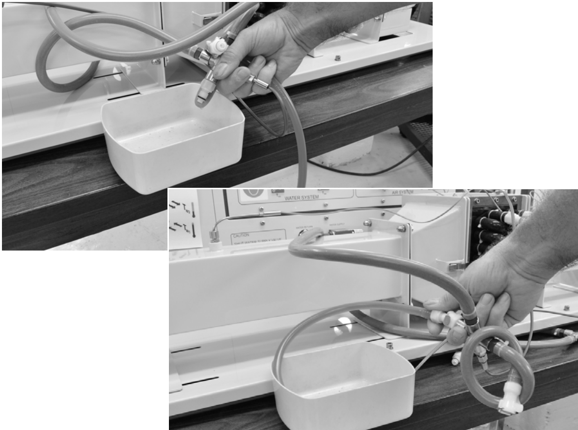
Figure 57 Drain the Water Pipes
