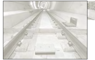
Track and Signalling Systems
