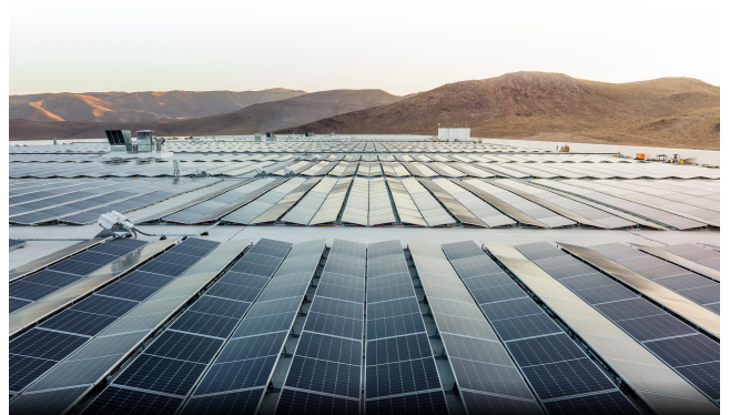
Solar Energy panel system
