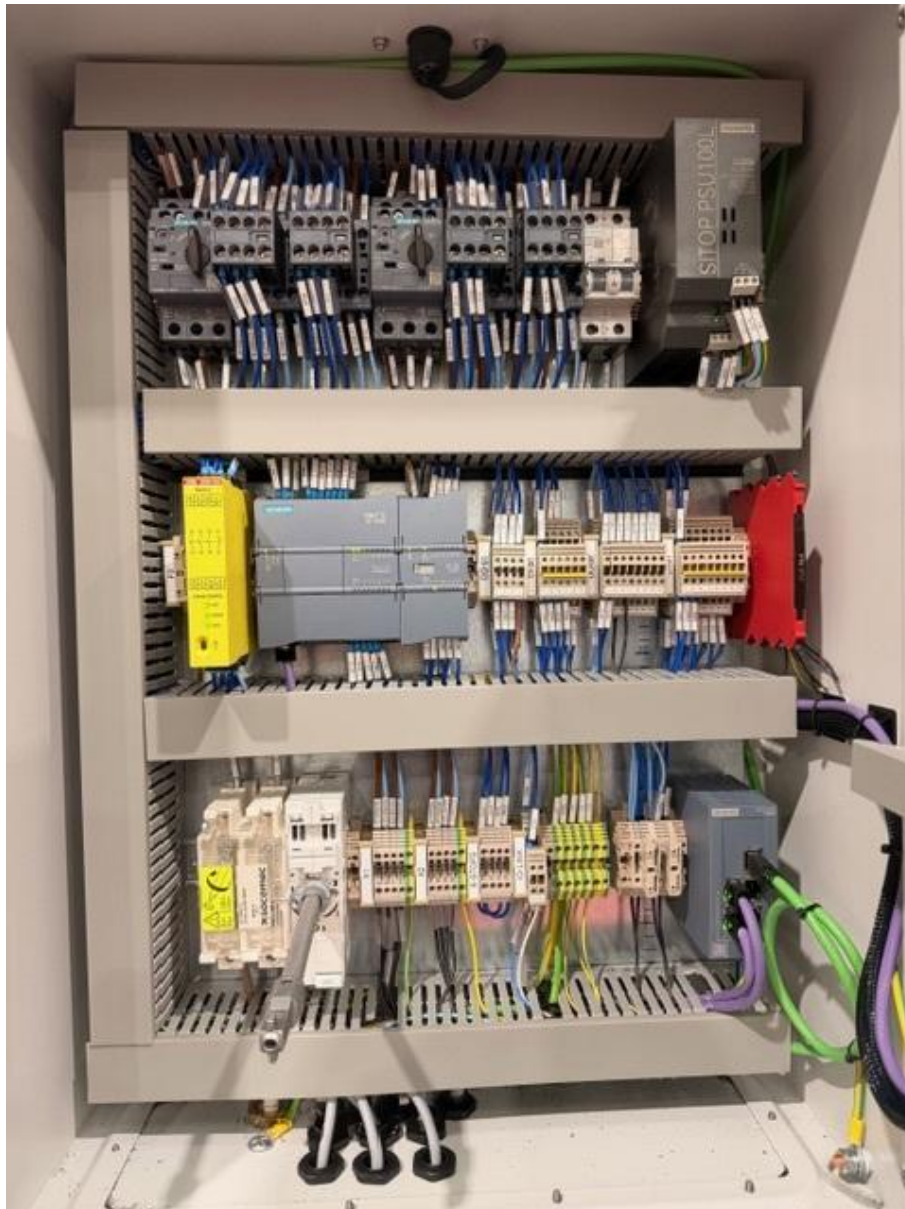
Figure 4 - Interior view of the panel showing all components.
