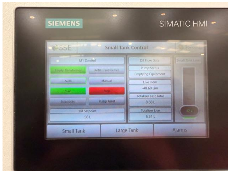
Figure 13 - Photo of HMI showing live flow data.
