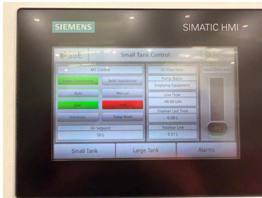
Figure 16 - Photo of HMI in normal operation.
