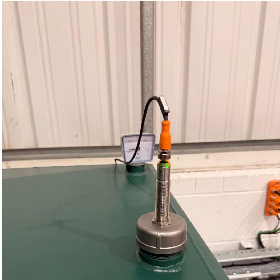
Figure 11 - IFM UGT813 level sensor installed on the transformer oil storage tank.
