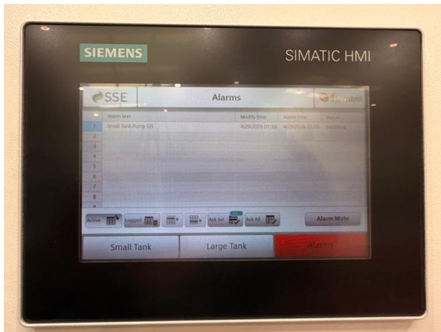
Figure 15 - HMI showing active alarms.
