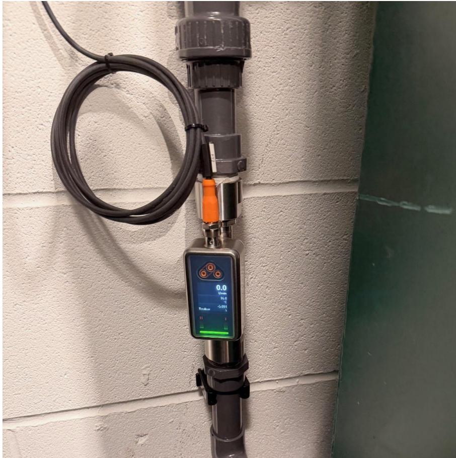
Figure 12 - IFM SU8030 clamp-on ultrasonic flow sensor installed on the 1" PVC transfer pipework.
