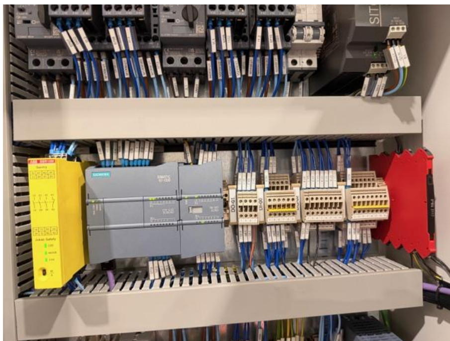
Figure 7 - Safety relay, PLC, input/output card and terminals.
