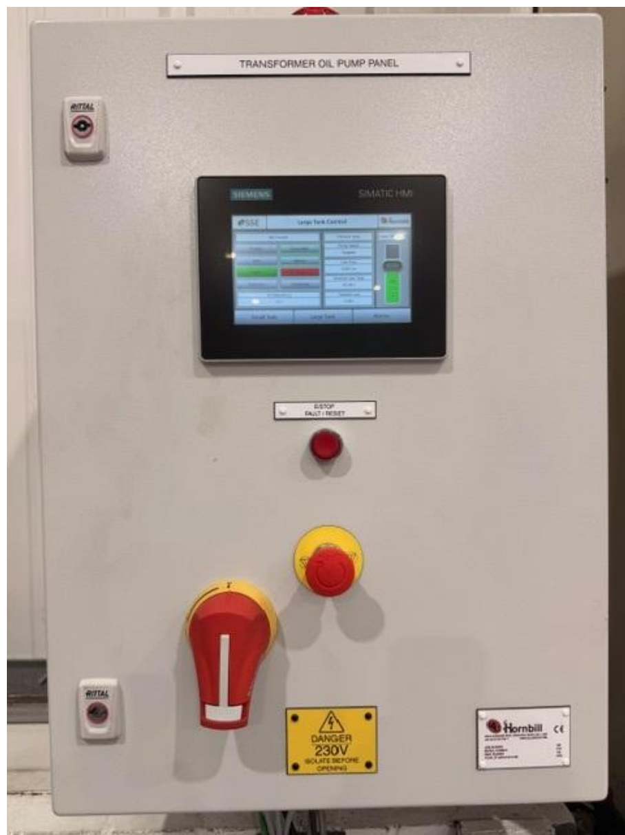
Figure 3 - Exterior view of the completed control panel.
