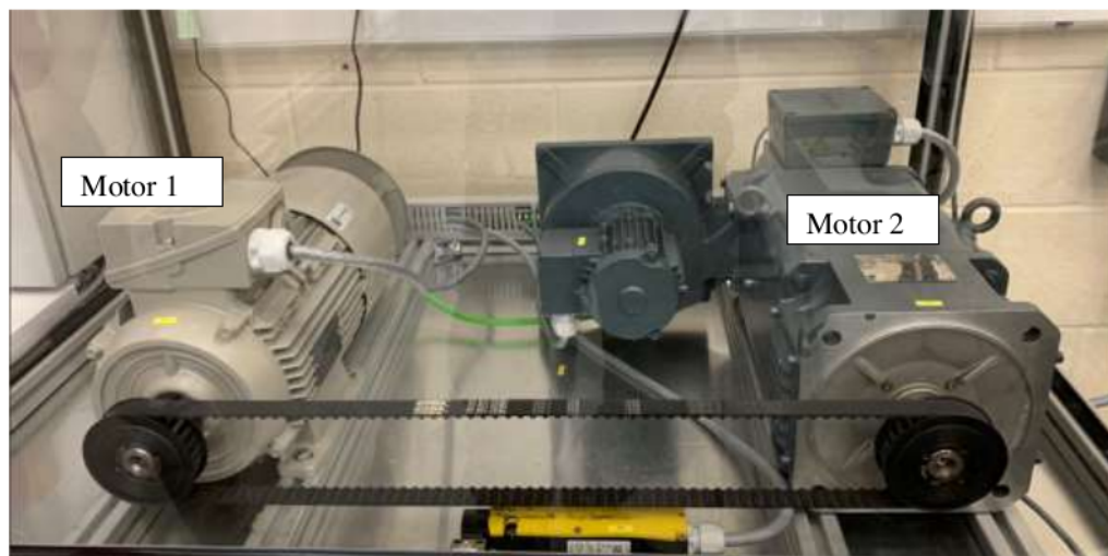
Figure 20 - Practical - Motor Setup
